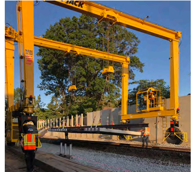
8. The PMT also planned for station infrastructure and platform work by having temporary platforms installed and using gangways to ensure the safe boarding and alighting of trains. These temporary platforms allowed the design-builder to perform all the necessary construction work at the stations, while protecting the public and avoiding disruption of train operations.
