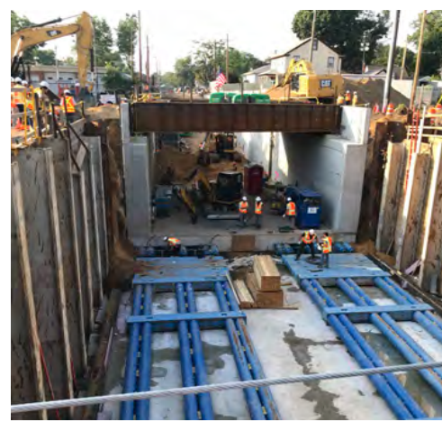
6. Box-jacking was used for the level crossing removals, with the entire bridge’s steel structure and concrete foundations fully constructed in a pit adjacent to the track
