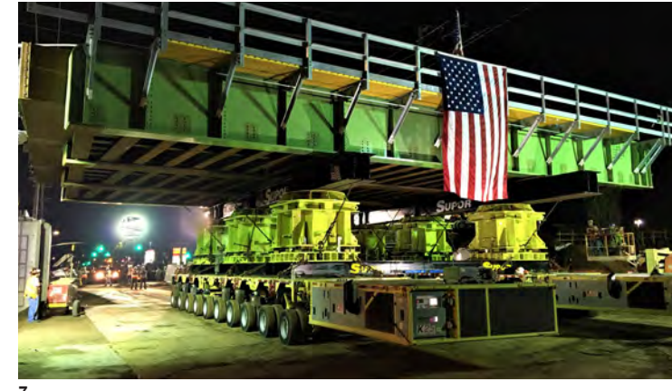
7. An SPMT (7), a steerable rolling gantry crane (8) and temporary platforms (9) were deployed to ensure continuous operation of the railway during works
