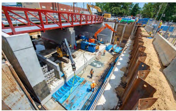
5. Box-jacking was used for the level crossing removals, with the entire bridge’s steel structure and concrete foundations fully constructed in a pit adjacent to the track
