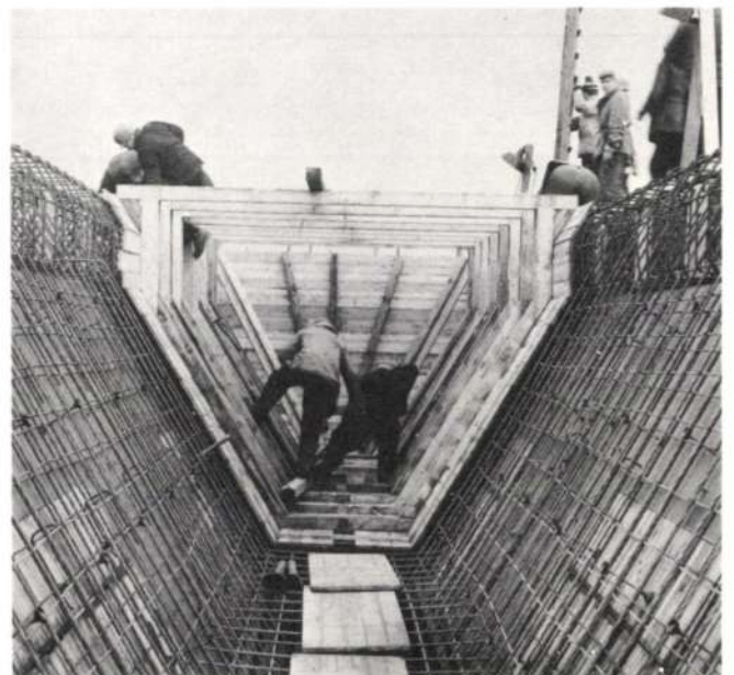
Fig. 5 Town Hall, Marl, W. Germany. Top shutter (reproduced with permission from Beton-und-Stahlbetonbau)
