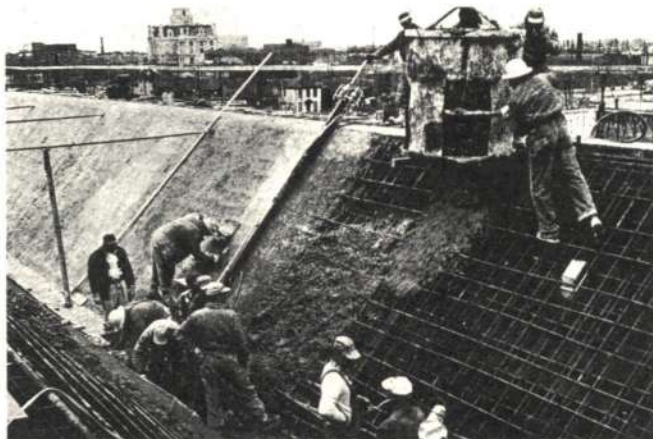
Fig. 10 57 ft. span post-stressed roof, Indiana State College (reproduced with permission from Engineering News Record)
