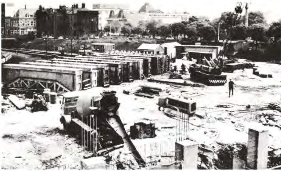
Fig. 7 Precasting portal beams on site. The three columns in the foreground are ready to receive beams (Photo: Sam Price)
