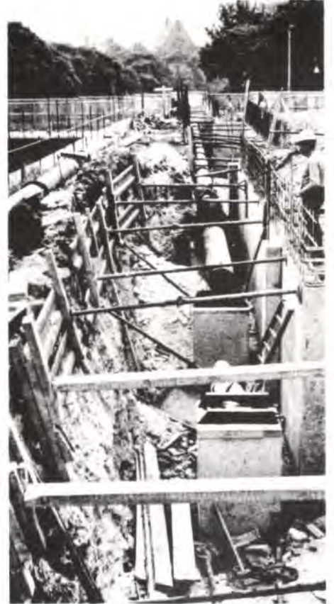
Fig. 5 Moving the seawater main. The old main is on the left, the new main being laid in parallel on new stools close to the back wall of the new car park (Photo: Sam Price)
