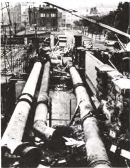
Fig. 11 above Burdon Road Bridge services. From the left : new water main, new gas main, old water main (Photo : George Curry of John Laing & Sons Ltd.)
