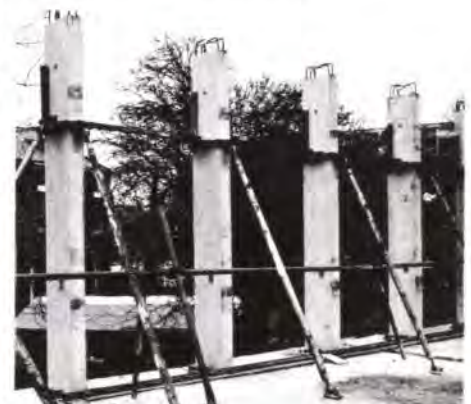
Fig. 17 below Precast mullions in an erection jig (Photo: John A. Herring, Sunderland)
