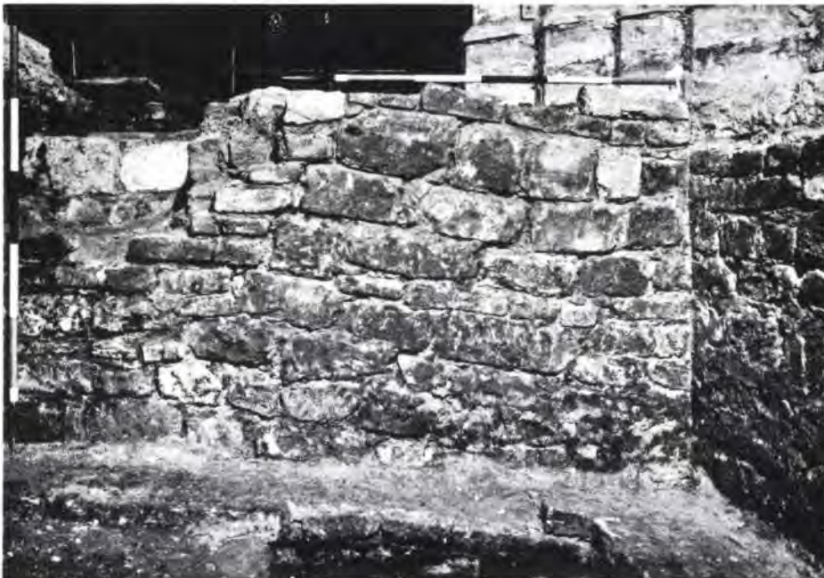
Fig. 5 Distortions in Norman walls below present floor level due to column on the right (Photo: by courtesy of the Royal Commission on Historic Monuments)
