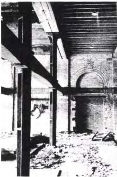
Fig. 13 above Fishbelly flanged beams for a mezzanine floor of 1855, inserted between the original cruciform columns of C warehouse (Photo: Malcolm Tucker)
