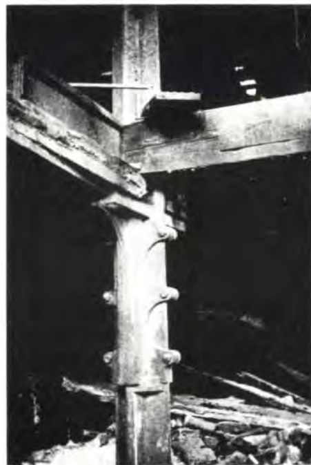
Fig. 14 below Cast iron clamp (c.1855) to support the later mezzanine floor (Photo: Malcolm Tucker)
