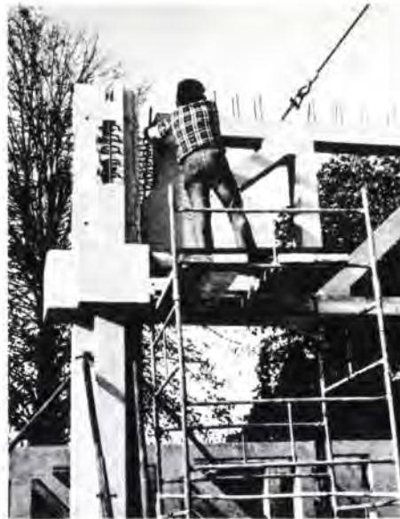
Fig. 6 Typical connection detail prior to concreting of truss to cruciform section column (Photo: Beecham Research Laboratories)
