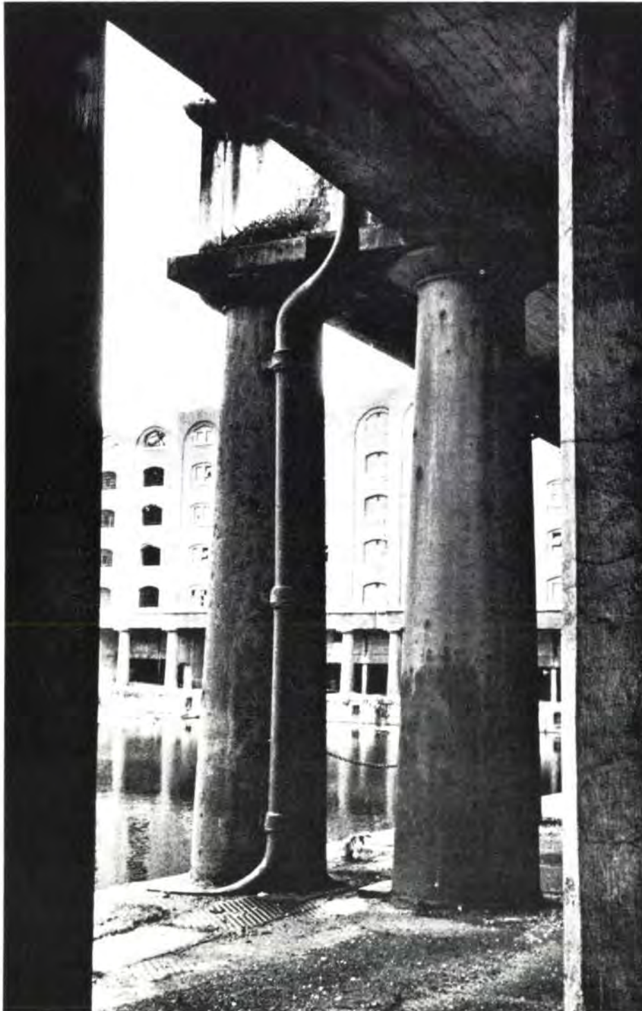
Fig. 5 Doric columns on the quay beneath B warehouse. Note rainwater drain pipe (Photo: Malcolm Tucker)
