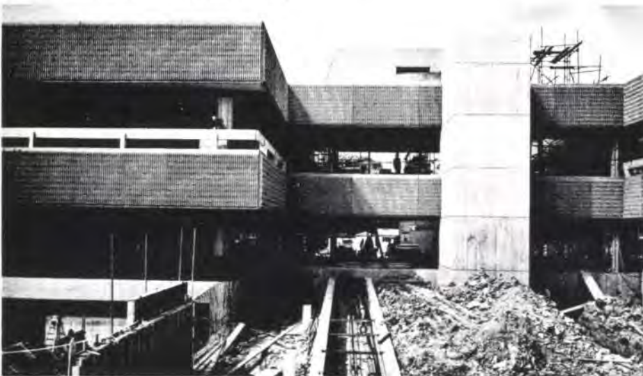
Fig. 8 In situ concrete link block between North & South Blocks Fascia panels are precast as for the main blocks (Photo: Beecham Research Laboratories)
