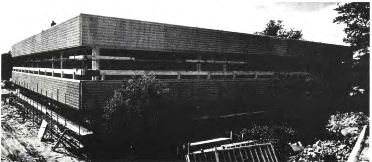
Fig. 9 North Block on completion of the structural frame (Photo: Beecham Research Laboratories)
