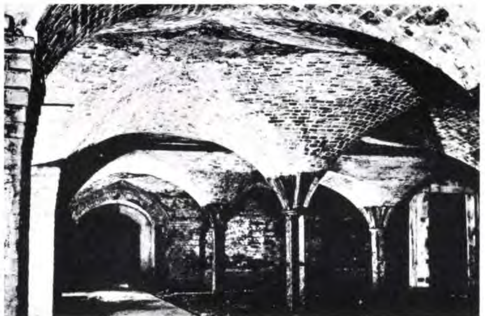
Fig. 9 below Groined vaults on cast iron columns under C warehouse (1828) (Photo : J. Flowerday)
