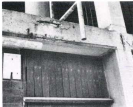
Fig. 9 Examples of spalling on the staircases (Cuthbert Harrowing House)
