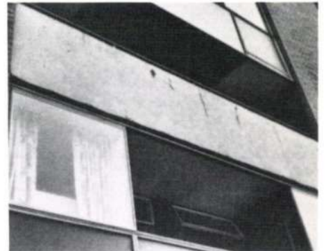
Fig. 10 Example of spalling on north facing access gallery (Bayer House)
