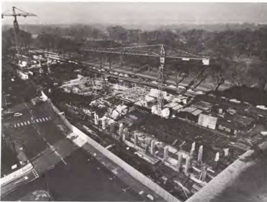
Fig. 3 Progress photo taken in December 1967 showing the awkward shape of the site (Photo: The contractors)
