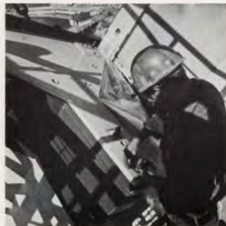
Fig. 34 Rib during erection. Grips for temporary anchorage being fitted (Photo: Max Dupain)
