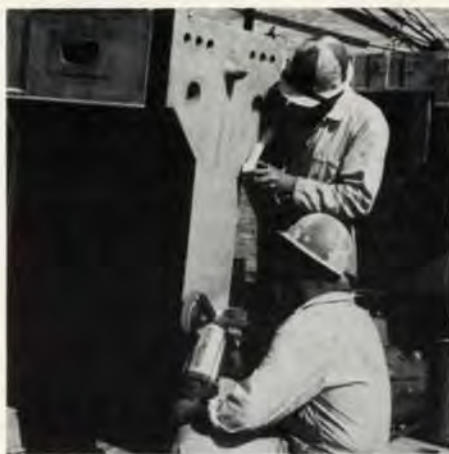
Fig. 1 Grinding the surface of a precast concrete rib segment prior to erection, and placing the masking polythene and tape (Photo: Max Dupain)
