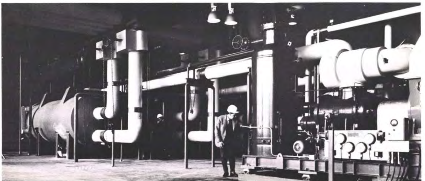
Below: The energy centre: first floor showing refrigeration equipment
