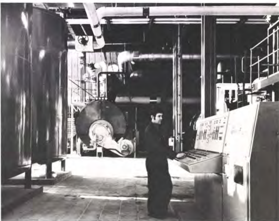
Below: Carbon dioxide recovery plant control panel. In the background is another of the boilers
