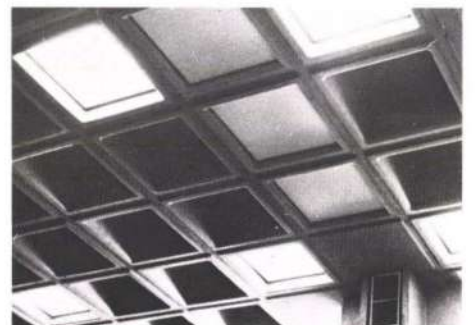
Fig. 22 Reference library - View of coffer ceiling showing coverings to air conditioning duct within coffers leading from a cruciform column
