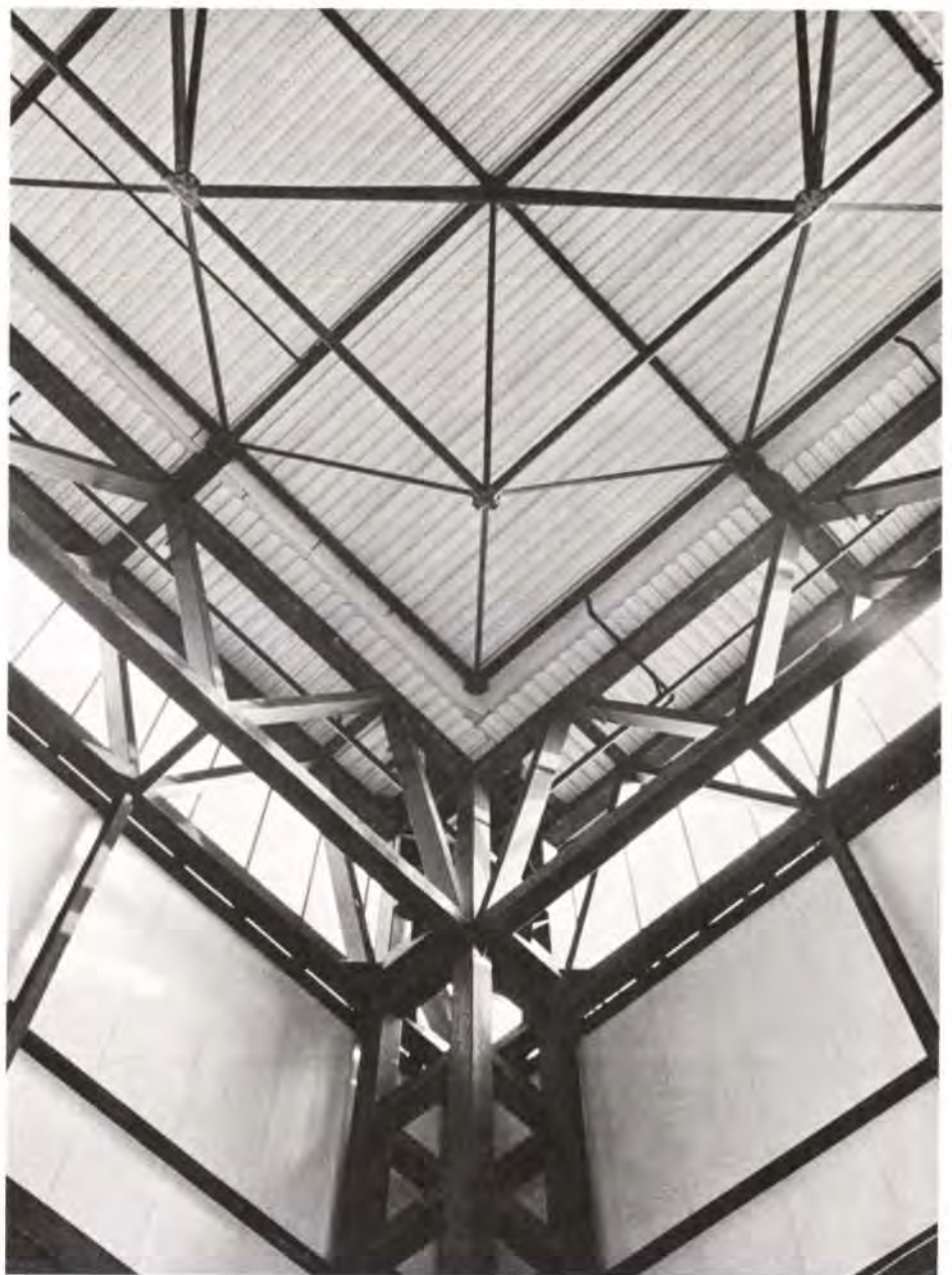
Fig. 2 View of the roof from a corner of an Exhibition Hall. (Photo: Harry Sowden)
