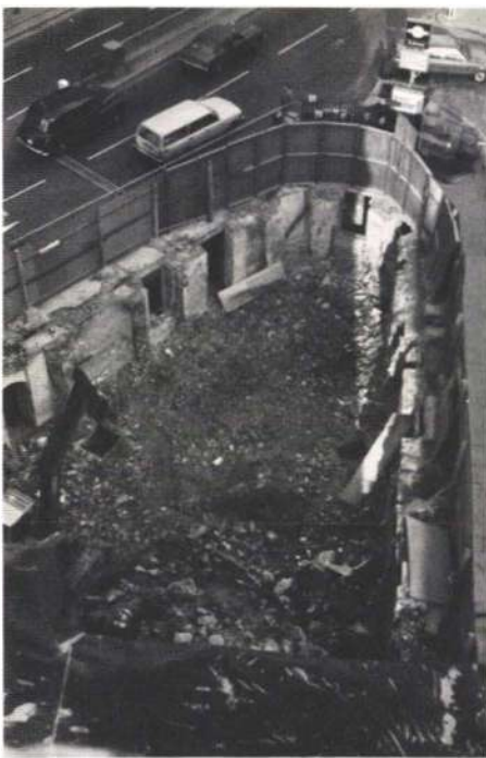
Fig. 5 Phase 2 site after demolition of fire station building in March 1976 (Photo: Michael Courtney)
