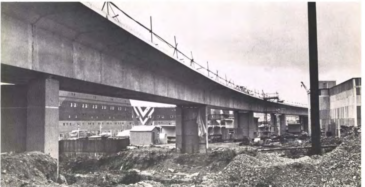
Fig. 9 Part of the viaduct on Byker Hill. The casting shed is on the right and the Byker Wall can be seen through the viaduct (Photo: Bill Smyth)
