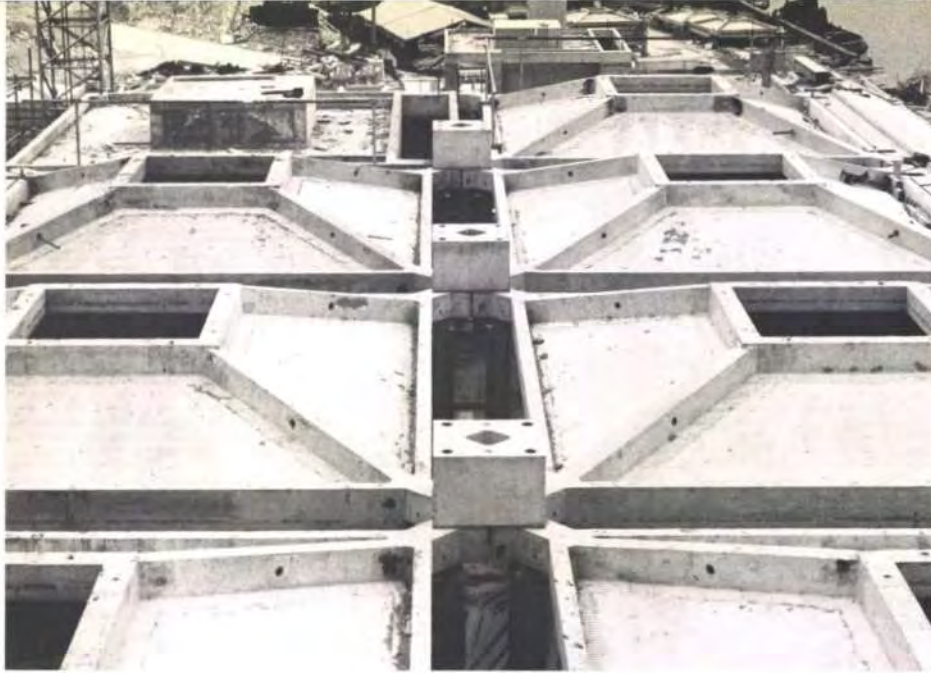
Fig. 23 Lloyd's Administrative Headquarters: 7.2 m bays with pyramids cast in one with four columns and no edge beams
