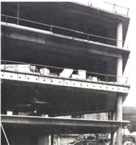
Fig. 6 Floor slabs of a typical module showing perimeter ventilation ducts being installed (Photo: A. L. Hunter)
