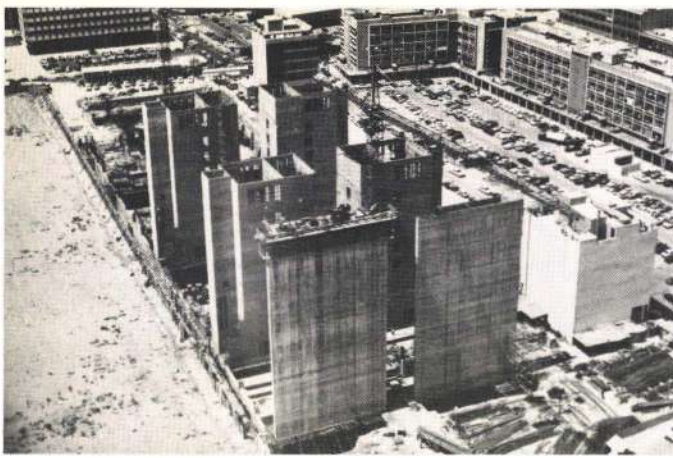
Fig. 7 The general site layout, with six slipformed cores cast and six still to be cast (Photo: Oscar Matri, Kuwait)
