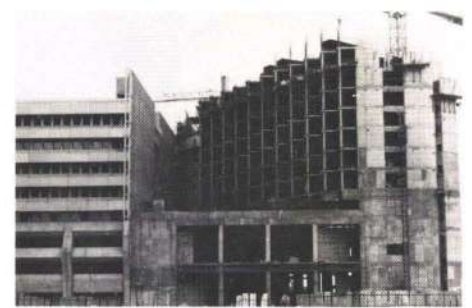
Fig. 9 South-west side of the hotel under construction, showing arrangement of bedroom windows, on 30 November 1978 (Photo: Oscar Matri, Kuwait)
