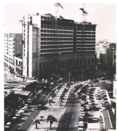
Fig. 6 The hotel under construction on 2 January 1979, with the Commercial Centre behind (Photo: Oscar Matri, Kuwait)
