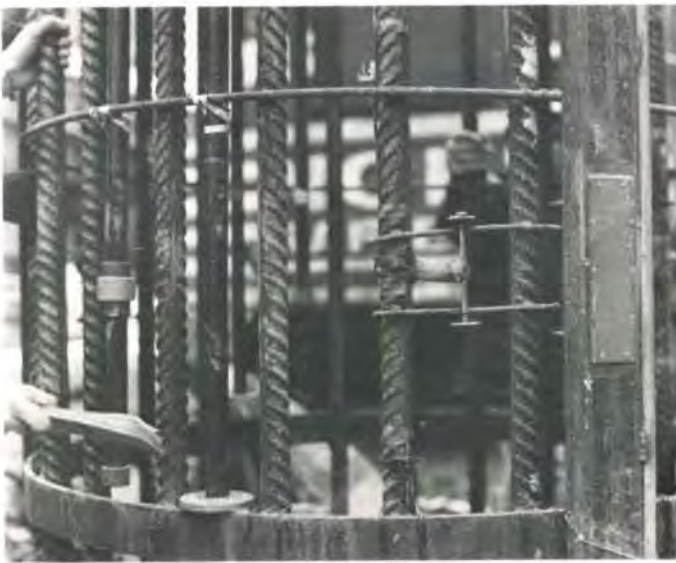
Fig. 7 Reinforcement cage showing, left to right, magnetic extensometer, rod extensometer, embedment strain gauge and vibrating wire strain gauge mounted inside box section (Photo: Frank Gadd)
