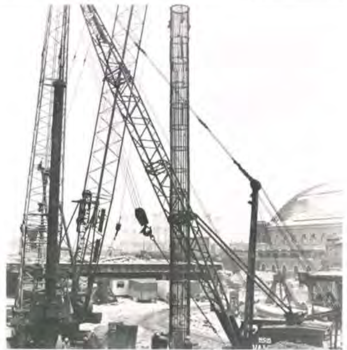
Fig. 4 Cage for 1.5 m diameter test pile being lifted from the 'rat-hole' (Photo: Frank Gadd)
