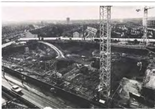
Fig. 6 General view of site showing sheet piles which are retained by ground anchors (Photo: John Laing & Son Ltd.)
