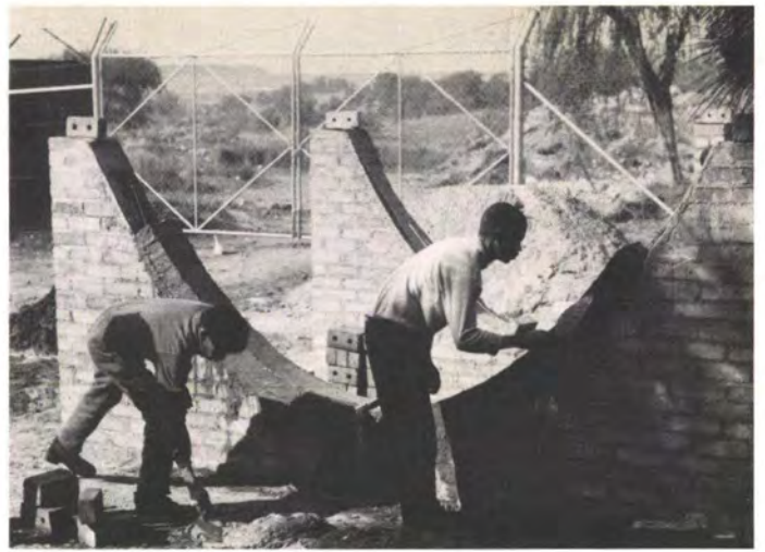
Fig. 5f Low-cost housing : fabricating the brick vault ribs, in two halves, on brick moulds
