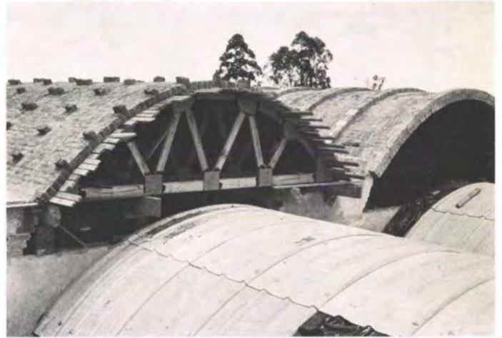
Fig. 6b Monis Winery : step in roof (Photo : Ove Arup & Partners, Zimbabwe)
