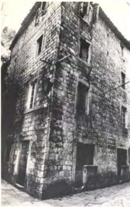
Fig. 6 Typical example of minor damage at Kotor
