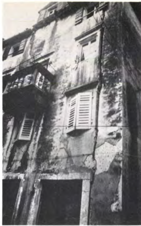
Fig. 4 Kotor: crack following straight joint between stone window surround and corner masonry
