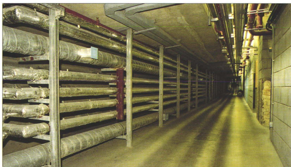
11. Left: Part of the building management system in the chiller plantroom.
