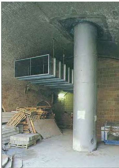
19. One of the building's permanent columns where it passes through the vault roof.
