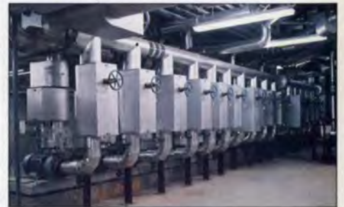
22. Secondary system pump sets.
