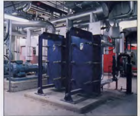
21. District heating heat exchangers.
