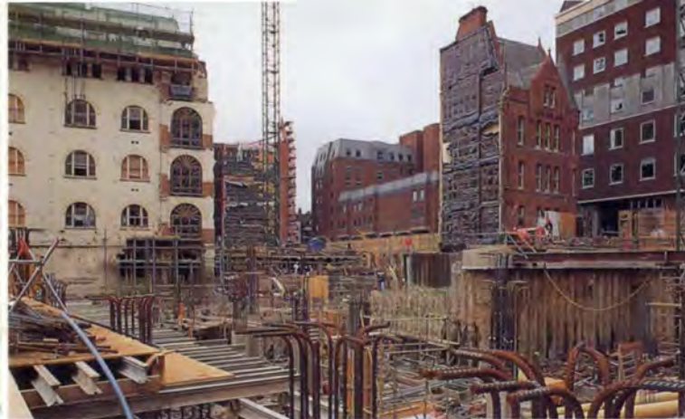
12. Basement excavation at September 1990. The retained building on the left forms the south side of the main atrium. On the right is the retained 'Jewel', with secant pile walling in its foreground.
