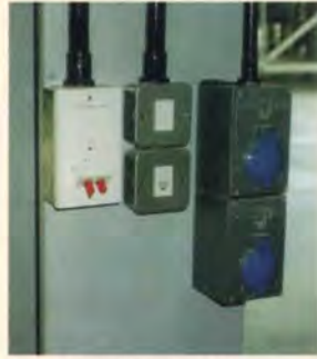
A. Fibre (left), voice (above centre) and data (below centre) terminations in hangar bay, with heavy duty power socket on the right.
