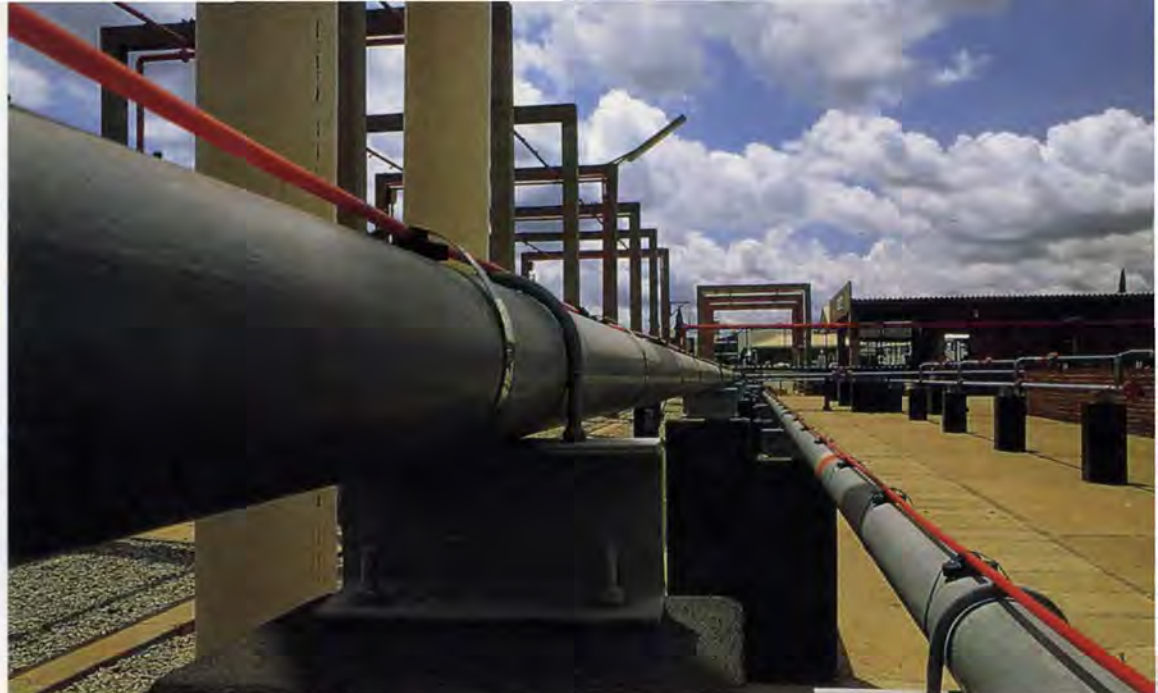
▲ 5. LPG pipes with check-fire tubing.
