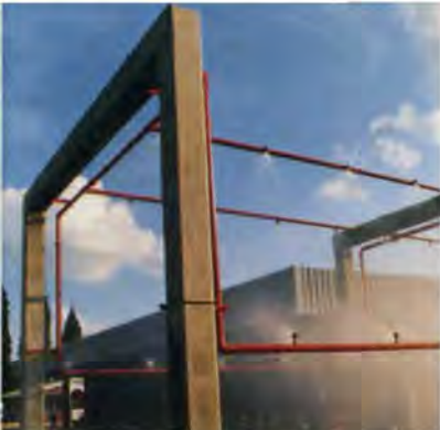
▲ 3. Road and rail area sprinklers.
