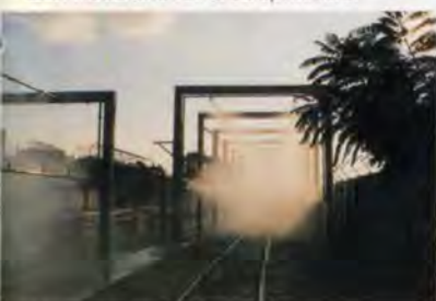
▲ 4. Rail decanting area sprinklers.
