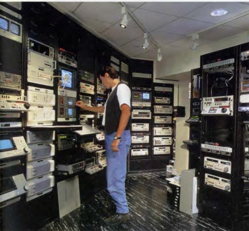
18. Video post-production facility: the Telecine Equipment Room
