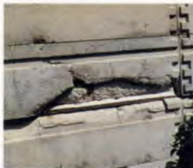
7. Blocks are stack-bonded without mortared joints. Reinforcement is horizontal and vertical in edge grooves, grouted with a fluid cement mortar. Rusting has led to spalling.
