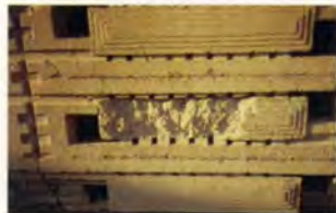
6. The original blocks are weak and friable, with high moisture movement due to absence of coarse aggregate. Wetting and drying can lead to surface breakdown.
