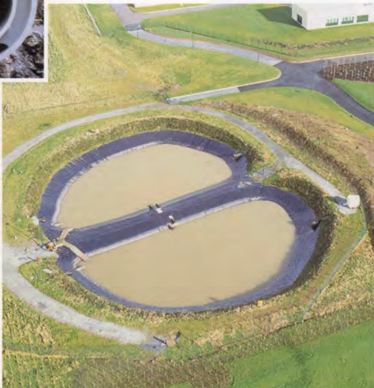
12. Completed retention pond: this acts as a catch basin for all storm/fire-water run-off.
