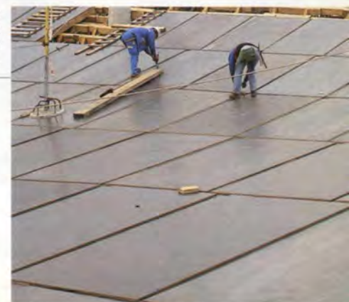
8. Right: Articulating modular formwork panels being assembled for the Zenith gallery floor slab.
