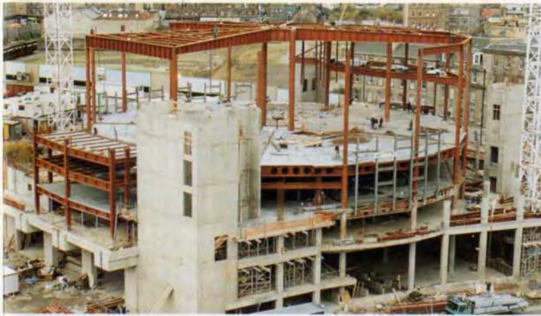
11. Progress on site by November 1993, showing the steel structure of the auditorium drum:
