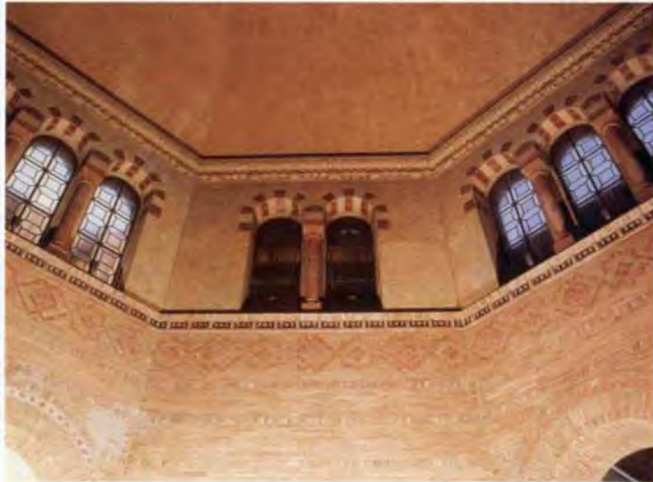
6. Rotunda brickwork: shotcrete strengthening was concealed in the corner piers behind the plaster and brick.
