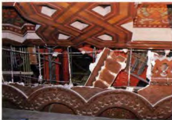
A. Ceiling damage from the Northridge earthquake
