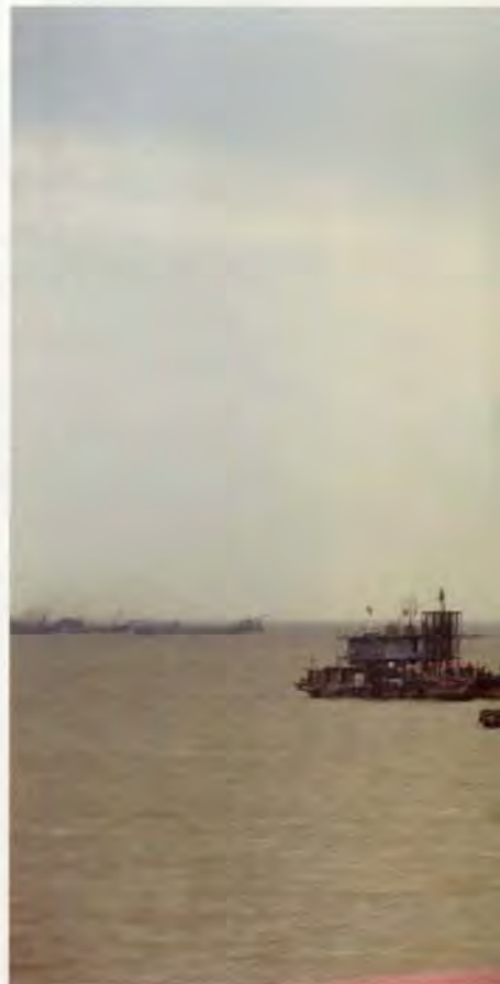
14. Placing jetty caissons: those in front of the crane to the right are temporarily stored, hence the angle.
