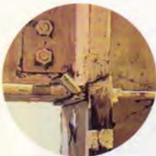
5. 'Pre-Northridge' moment connection: Fracture through column flange.
