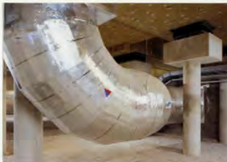
5. Foundation column with spring on pile cap (right). On the left is one of the undercroft air ducts.
