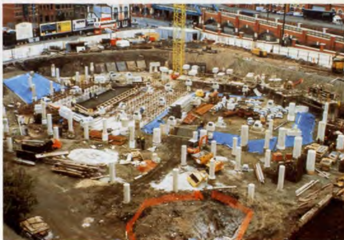
6. The site, looking west, in October 1993. Some columns already have caps and spring bearings in place.
