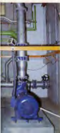
14. Utility pool variable speed main pump and standby 594m 3 /hr.
