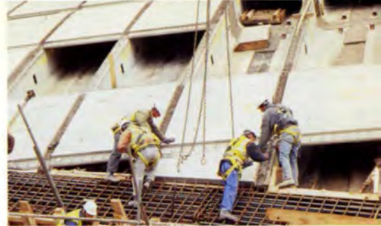
6. Shell roof detail showing lower T precast units, upper precast roof units.
