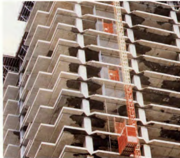
7. 100MPa high strength concrete structure at Taikoo Shing City Plaza, Hong Kong.
