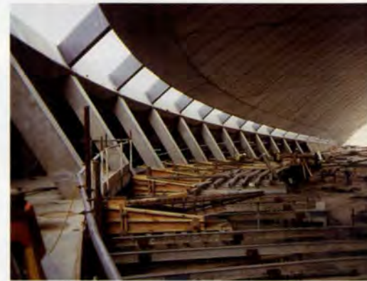
23. South-east side: shell supported by variable length steel arms through the lighting slot.
