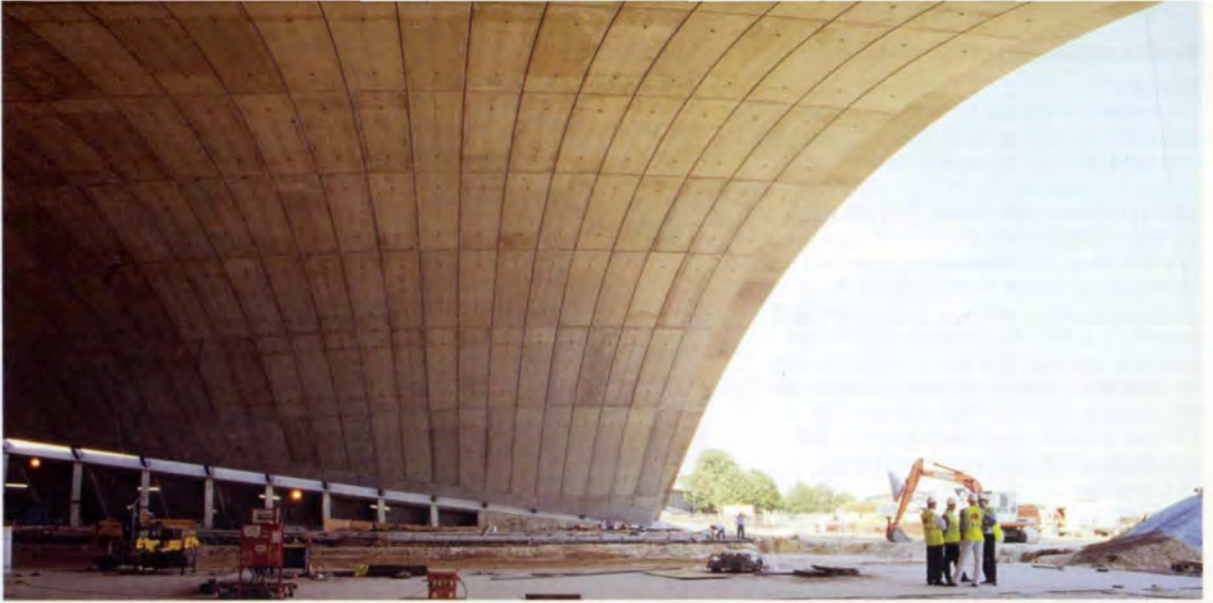
15. The shell at the topping out ceremony, July 1996. The perimeter light slot is visible, starting from the front foundations and increasing in width as it moves to the rear of the shell.
