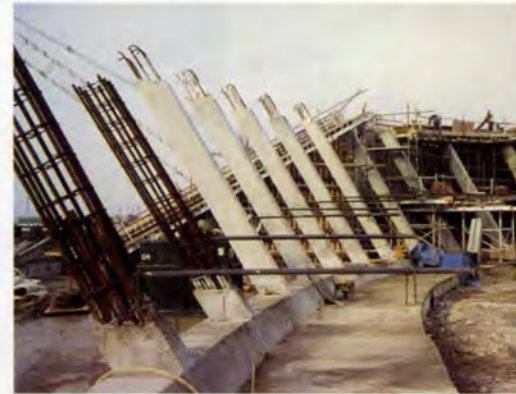
22. South-east side: inclined columns supporting the lower in situ edge beam at abutment level.
