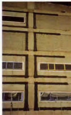
14a. Blockwork jointing at the south end of the Wall. The black stripes are the flexible waterproofing installed across 40mm movement joints prior to application of waterproof membrane across whole Wall.
