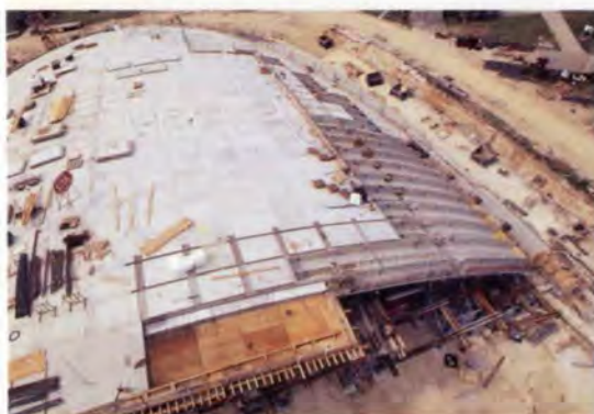
12. Aerial view of the nearly completed shell. Formwork for the in situ canopy in the foreground, June 1996.
