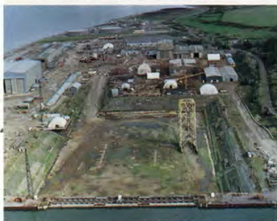
2. Nigg dry dock looking north before the start of the refurbishment works.
