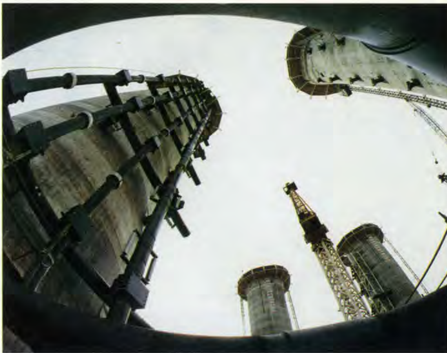
8. Exterior pipework on shafts.
