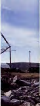
14 Right. Modified entrance ramp with rock armoured side slopes. The Lampson can be seen lifting a redundant 800 tonne crane base from the dock in background.
