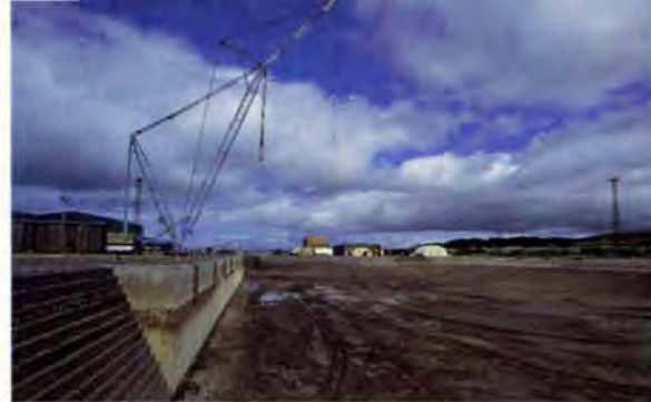
13 Left. Completed refurbishment works with the Lampson crane sitting on top of the new wall.
