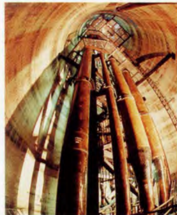
7. GRE pipework for oil storage system inside substructure.
