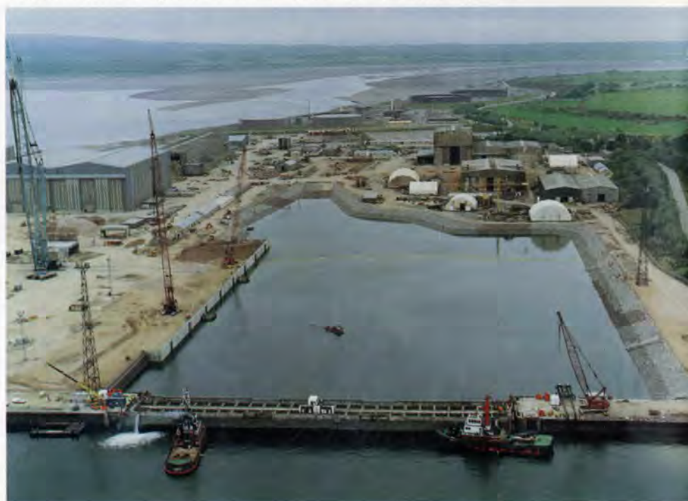
3. Dry dock flooded following completion of the new quay wall (left in picture) and slope works.
