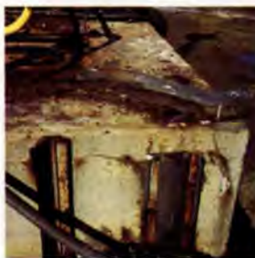
16. Existing lip and caisson seals on the quoin of the west roundhead.
