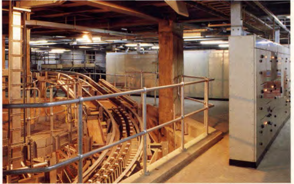
3. The top of the spiral at Terminal 1, showing automated control panels.
