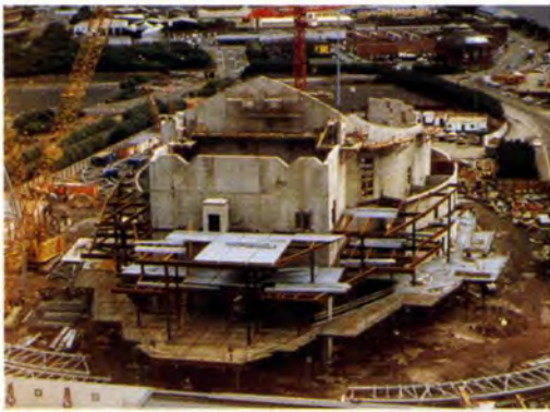
8. Concrete walls complete, floor plates wrapping around walls, and arches about to be erected.
