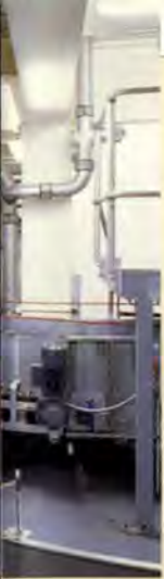
7. Conveyor systems at mezzanine in Terminal 4, showing co-ordination of building, services, and automation, and X-ray screening equipment.
