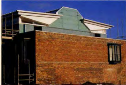
9. The condenser's location, behind the louvres.
