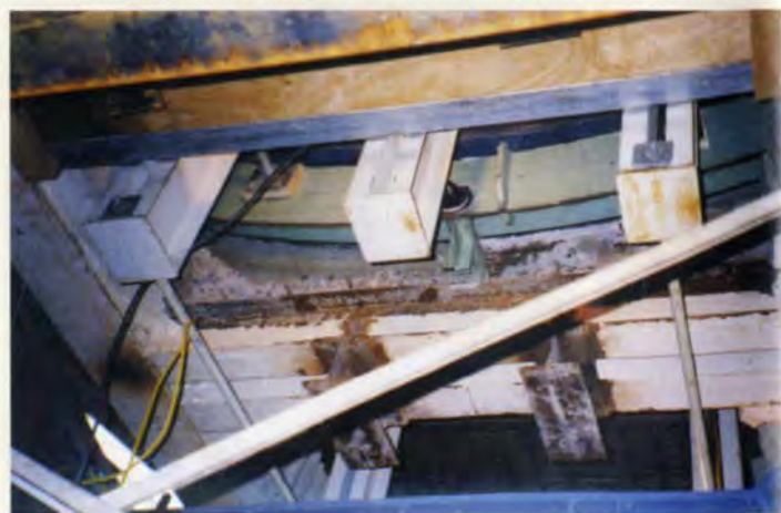
12. The disc still supported by the existing structure after being raised. The three vertical beams are part of the grillage. The new structure is installed below, ready for load transfer of the disc.
