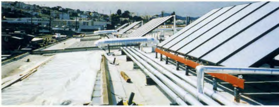
6. Solar panels and skylights on the roof.
