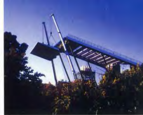
16. Cantilevered tip of Forest Gallery canopy being dual crane lifted into position.
