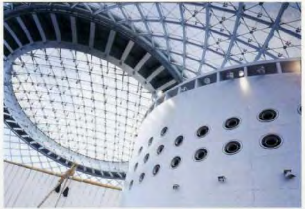
14. Close up of ring beam and core structure (note ventilation ducts on the wall)
