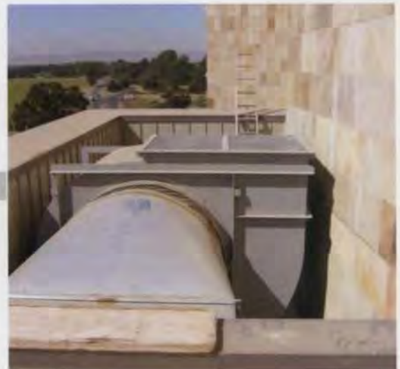
18. Lobby smoke exhaust fan.
