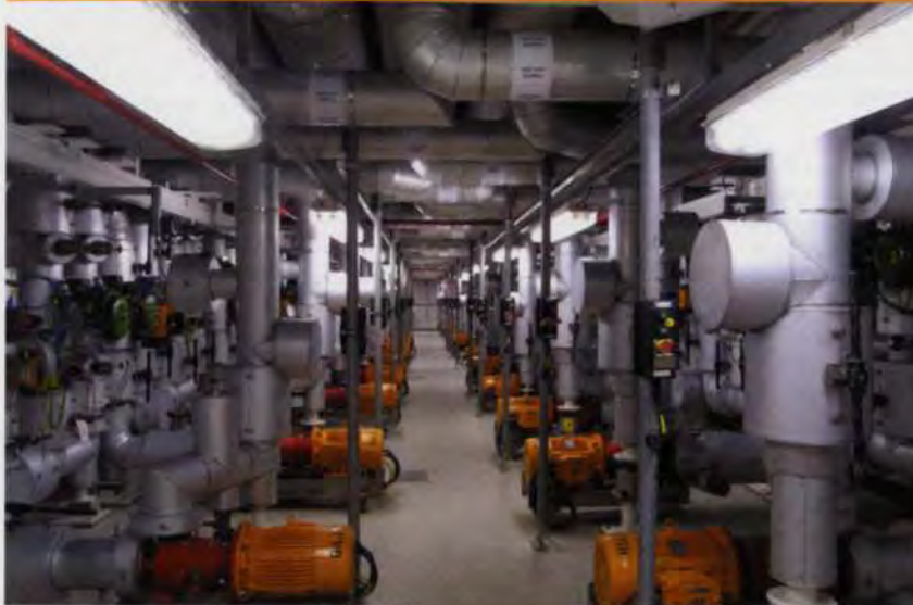
20. Jacket pump room in the production building.
