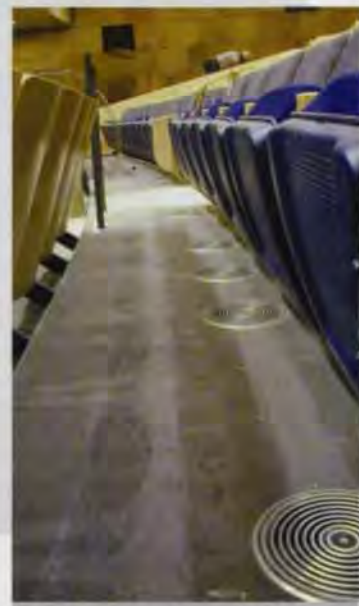
13. Jackson Hall floor diffusers.
