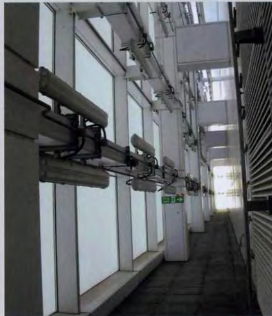
7. Crown lighting (at roof levels 43/44) for the HSBC symbol.
