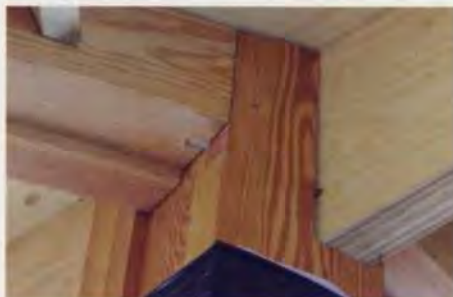
4 above. Connection detail between rafter, Douglas Fir column, and Kerto primary beam.
