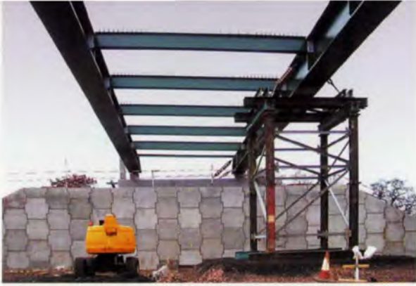
8. Simple, consistent design and construction: typical ladder beam deck and reinforced earth end-supports for two-span overbridges.
