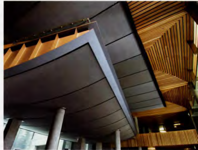
9. The 16m square mezzanine connects to the concrete columns through steel collars and dowels.
