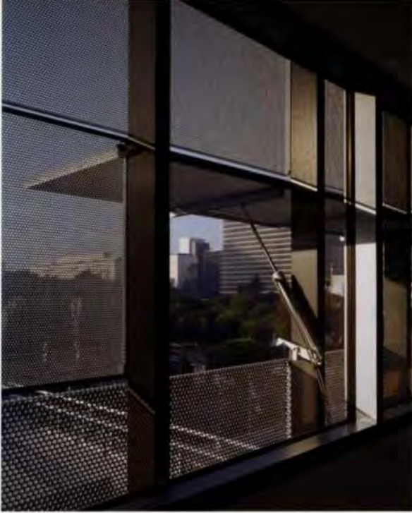
3. Interior view from office of scrim pneumatic actuators.
