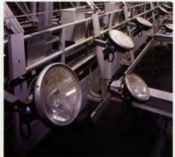
9. Typical floodlighting units.
