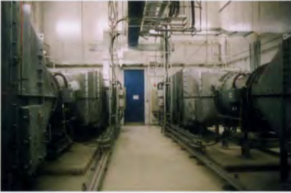
9. Tunnel ventilation plant.
