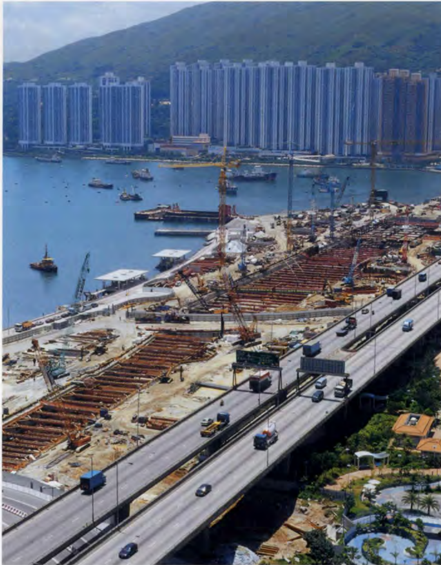
18. The Tsuen Wan bypass elevated highway runs along the north-east side of the site. The risk of the excavation works causing excessive ground movements that might affect the structure were mitigated at design stage by the choice of preloaded struts and by adjusting the railway alignment to bring the structure outside the zone of influence of the excavation.
