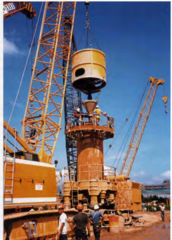
5. Large capacity rotator was used for pile casing installation and the subsequent casing extraction during concreting.
