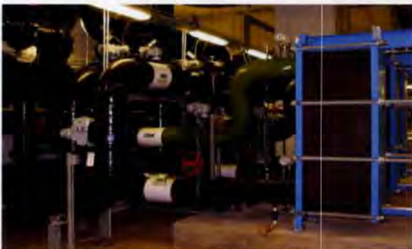
7. Plate heat exchanger and pipework from seawater pumping station in main station plantroom.
