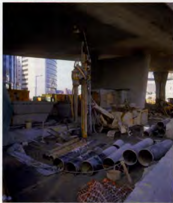
8. Specially adapted rig to install pipe piles below the Hung Hom bypass.
