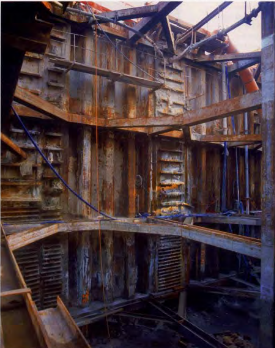
9. The maximum four levels of struts at the western end of the excavation.
