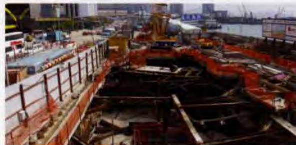
7. Gas governor (behind hoarding on the left) and temporary support for cross-harbour gas mains.
