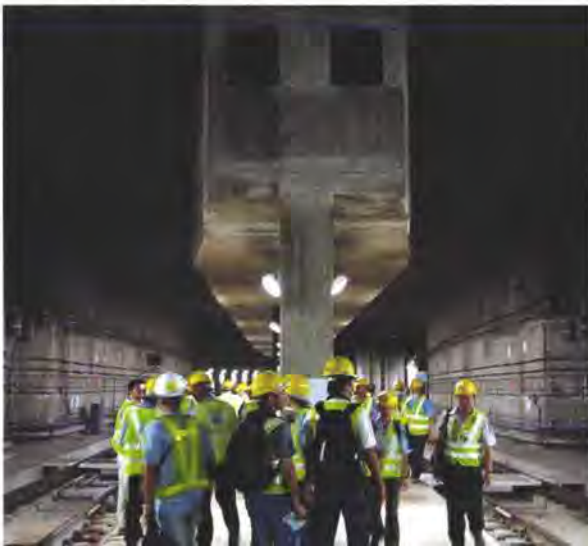
3. View of concrete air ducts supplying tunnel cooling to the twin-track tunnel.
