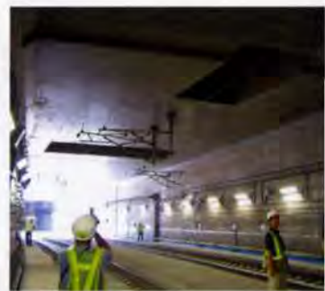
14. Smoke extracted before it can enter Hung Hom station.
