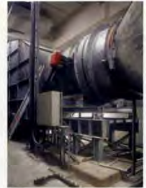
10. Tunnel ventilation fan in station.
