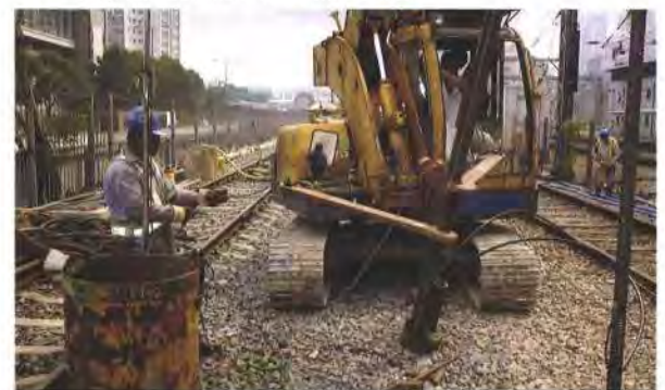
9. Minipile foundations being placed near live rails at the Ho Tung Lau maintenance centre site A.
