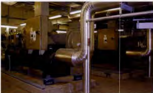
6. Water-cooled centrifugal chiller in main station plantroom.
