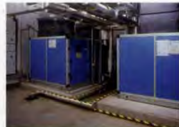
11. Tunnel cooling air-handling unit in station.
