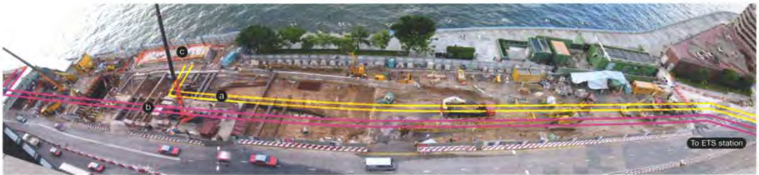
8. East Tsim Sha Tsui promenade, showing the running tunnel site with (a) intake pipes, (b) outfall pipes and (c) the new seawater pumping station.
