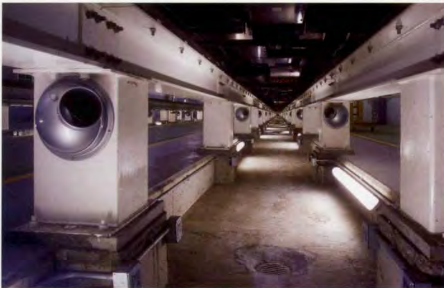
4. Spot cooling ducts at low level.
