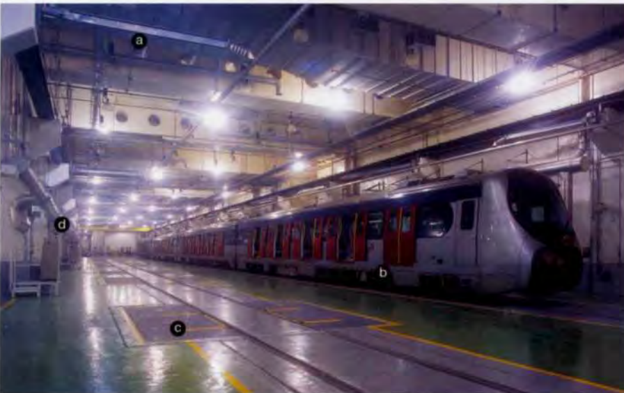
5. Heavy maintenance track - (a) retractable overhead line, (b) EMU, (c) underfloor lifting pit, (d) Spot cooling ducts.
