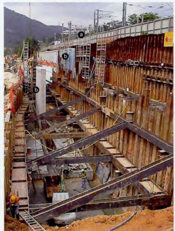
12. Temporary excavation support adjacent to East Rail - (a) East Rail, (b) retaining walls under construction.
