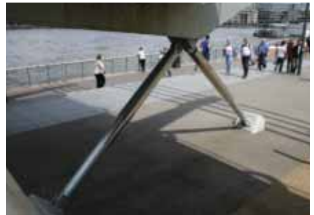
9. Diagonally braced viscous damper under abutment.
