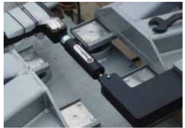
8. Viscous damper under bridge deck.
