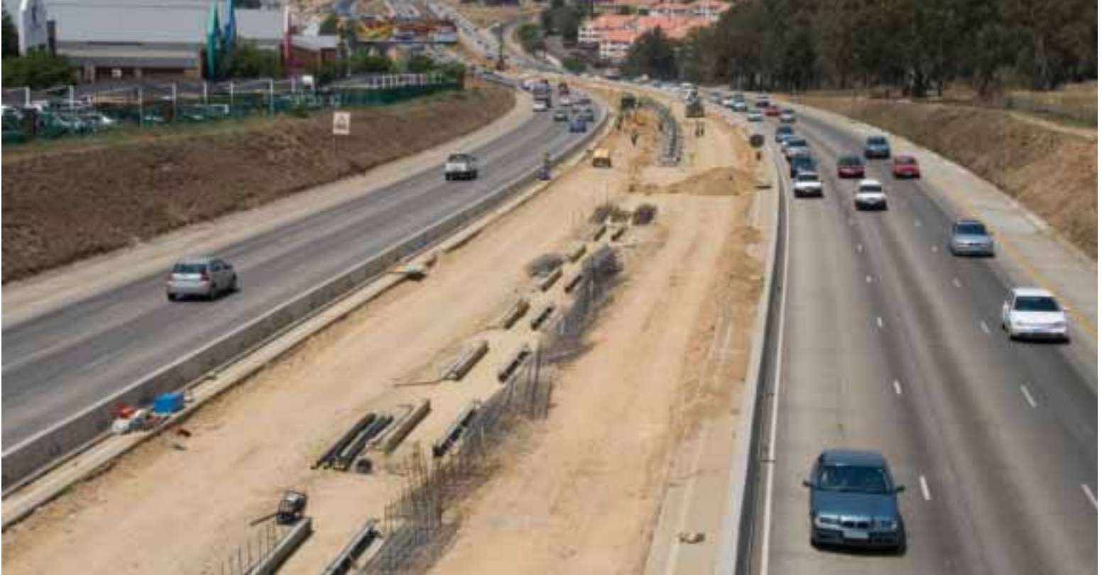
10. The Gauteng Freeway Improvement Scheme: adding additional central lanes while maintaining full bidirectional flow.
