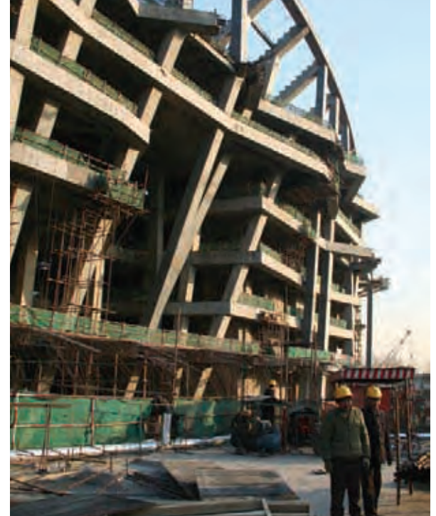
2. Columns are inclined both radially and circumferentially at the back of the bowl.
