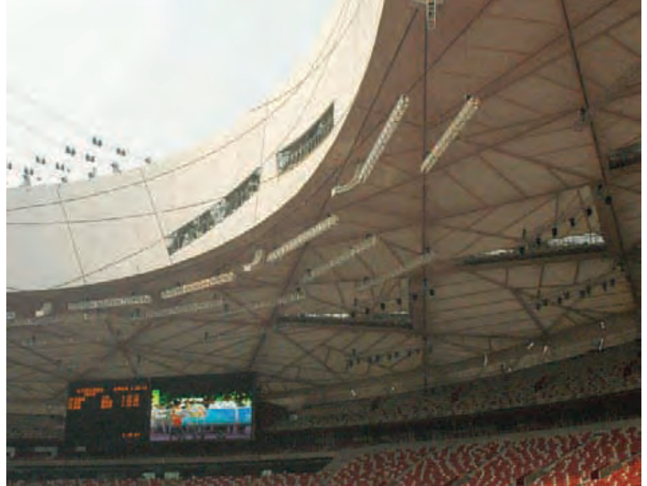
3. The inner membrane is a single-layer translucent PTFE membrane, which serves as the acoustic ceiling and provides shade for the spectators.
