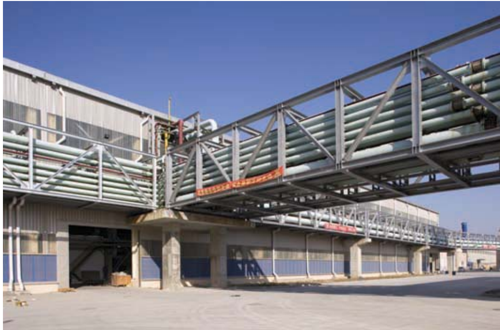
15. Pipe bridges accommodate the large quantity of process pipework, etc.
