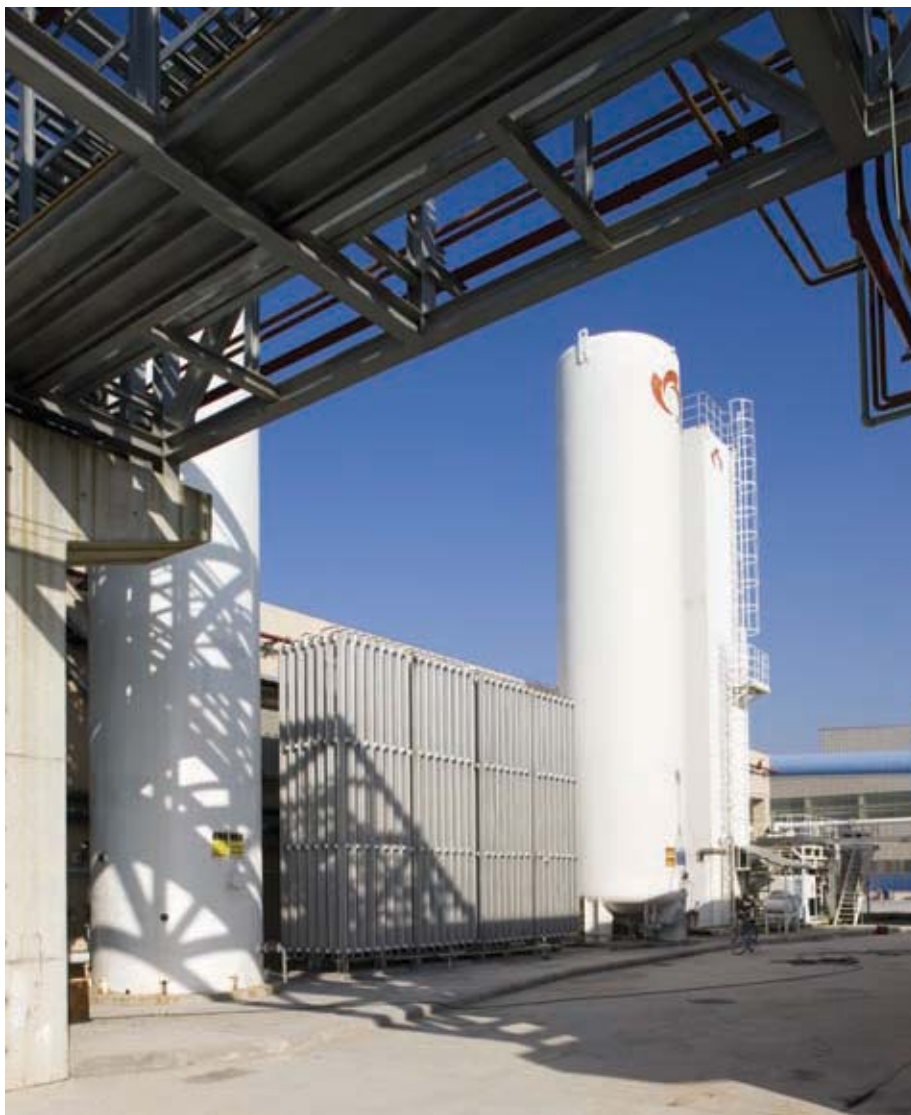
24. Nitrogen gas storage tanks.
