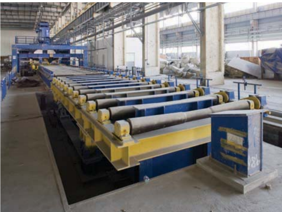
17. The effect of loading impact on machinery was critical to the foundation design.
