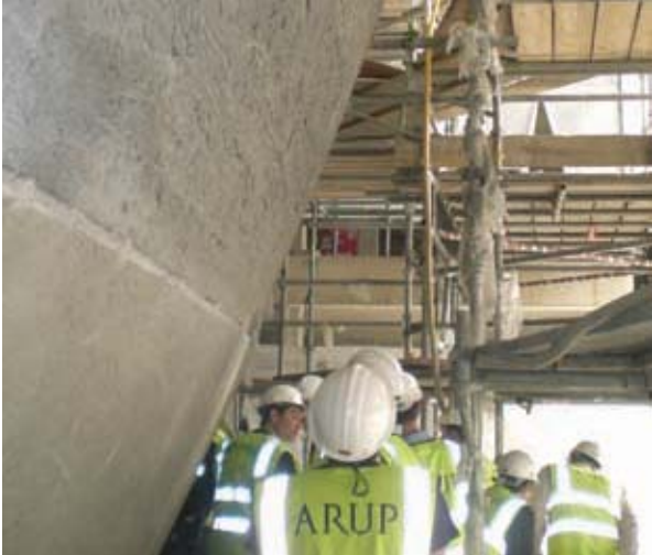
23. Finished surface of the wet sprayed concrete above, and the dry sprayed concrete below.
