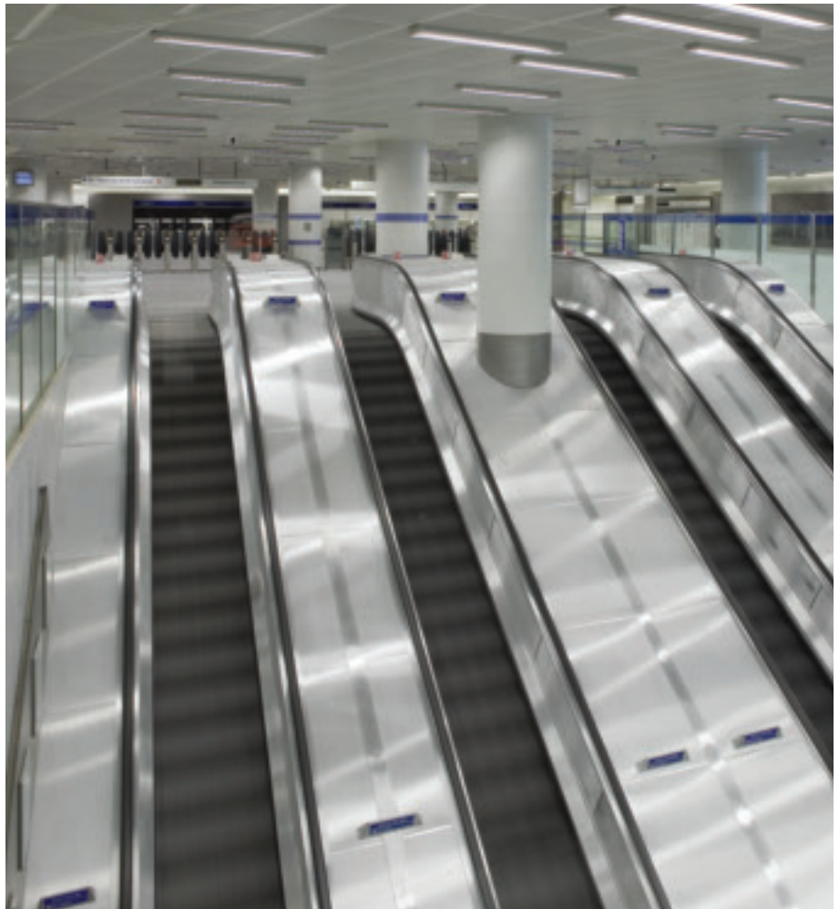
12. Escalators are the centrepiece of human movement in a wide range of public buildings and atria, and their safety record is impressive (above: King’s Cross St Pancras Underground).
