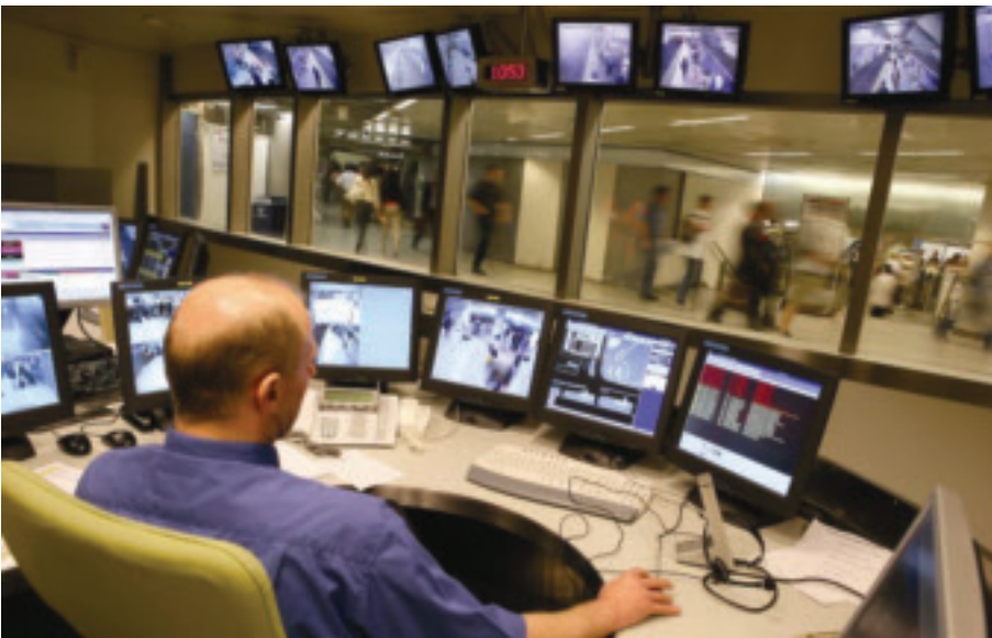
10. Control room at King's Cross St Pancras Underground station.
