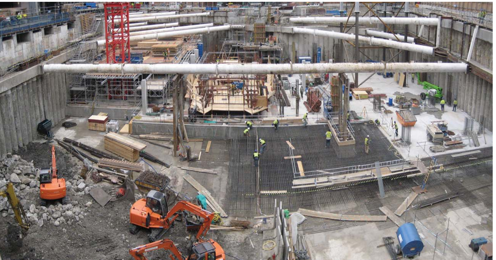
29. Site view to the south, showing slipform platform prepared for launch from the lower basement raft slab, between propped secant pile and existing buttress retaining walls.
