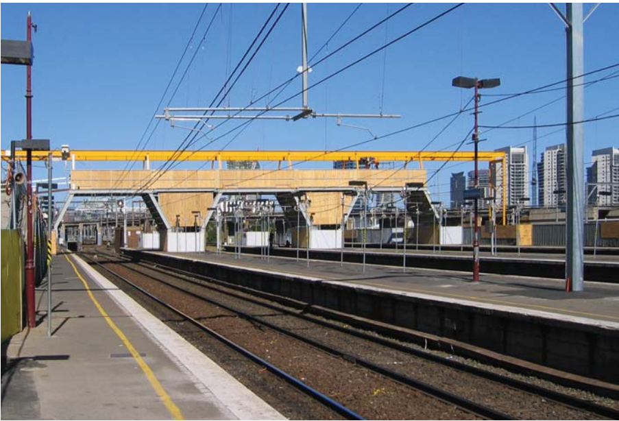
14. Erection of "crash deck" prior to any construction activity of the new concourse structures.
