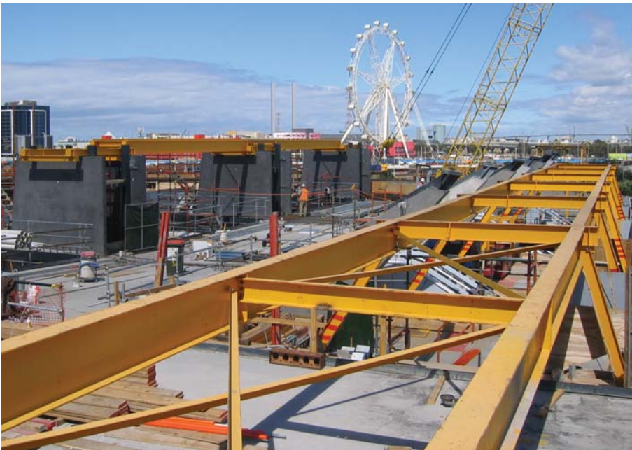
18. Crash deck and temporary roof skating structure viewed from the station embankment.
