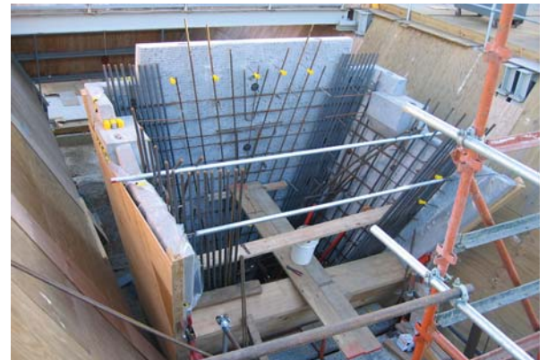
16. Pier precast elements erected and main reinforcement placed prior to in situ concrete pour.
