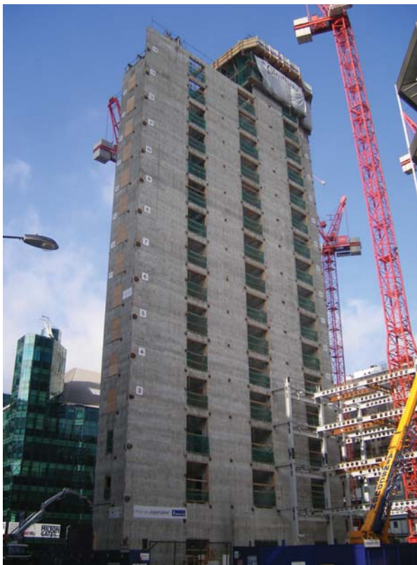
30. View from the south-east corner of slip-form core construction progressed to level 15 of 21, with the first four-storey bay of steelwork commenced.
