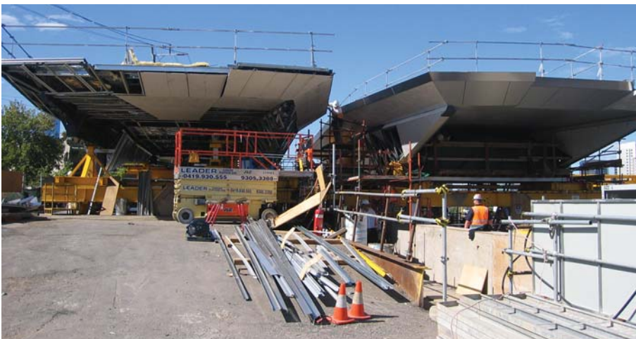
19. Concourse roofs assembled on top of the embankment, fully clad prior to skating into position.
