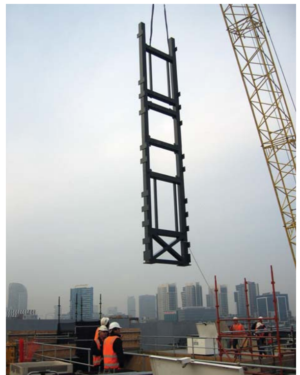
17. Lifting front lift shaft ladder frame across the rail tracks above the crash deck.
