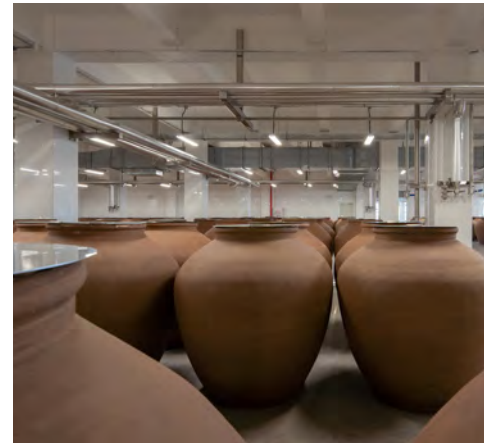
9: Vibration isolation bearings between columns and pile foundations in the wine storage blocks ensure the pottery jars used in the fermentation process are protected from seismic damage
