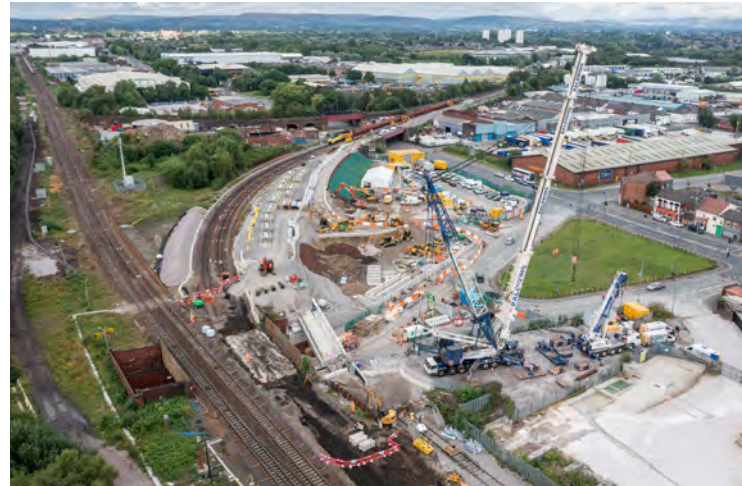
7: Changes to the track alignment on the route out of Manchester have boosted line speed by 42kph
