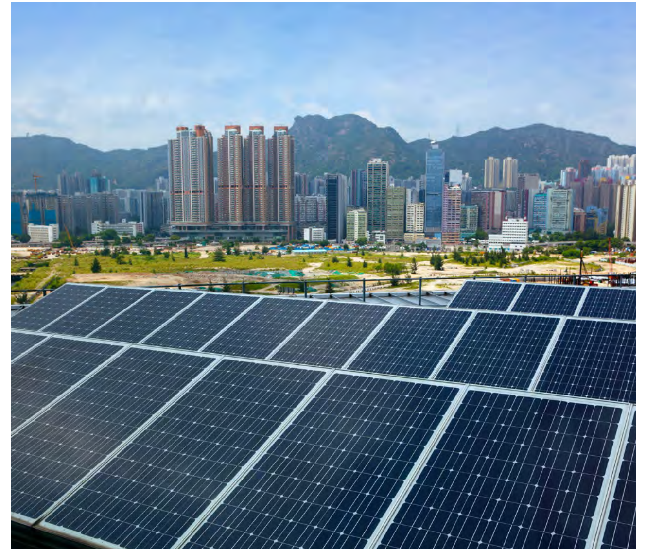
Rooftop solar panels at Kai Tak, Hong Kong
