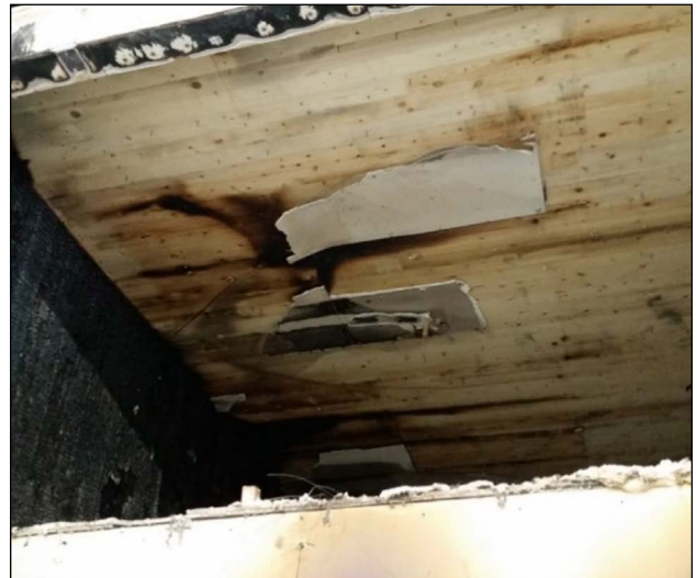
Figure 44: USFS-ICC - Test 3 – Post-test photo – living room ceiling
