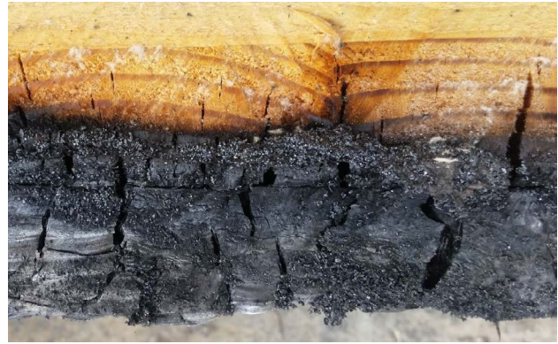
CLT panel post fire test with non-debonding adhesive
