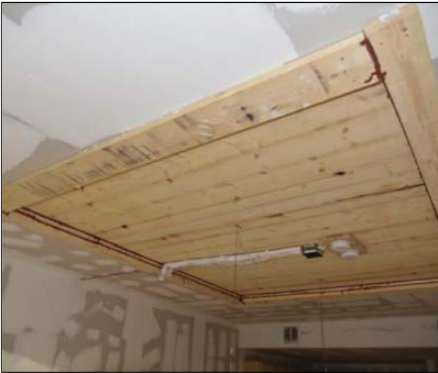
Figure 45: USFS-ICC Partially exposed ceiling in Test 2 (30% exposed) – Post-test photo
