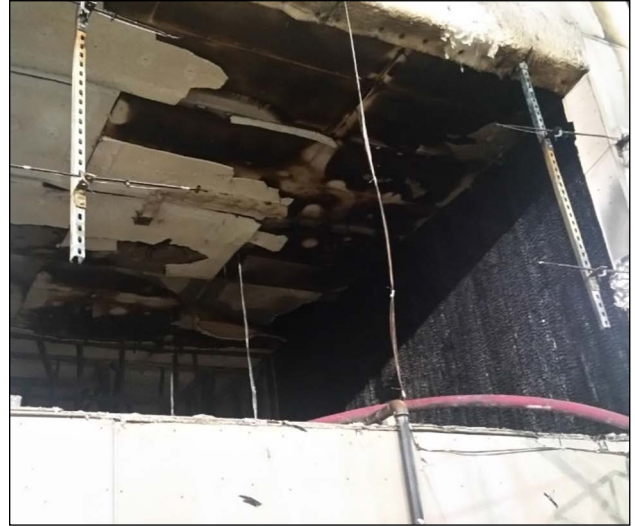
Figure 42: USFS-ICC – Test 3 – Post-test photo – bedroom ceiling
