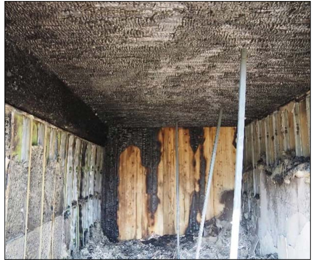
Figure 46: NRC 2023 Test 2 (100% ceiling exposed, post-test after removal of protection to rear wall)
