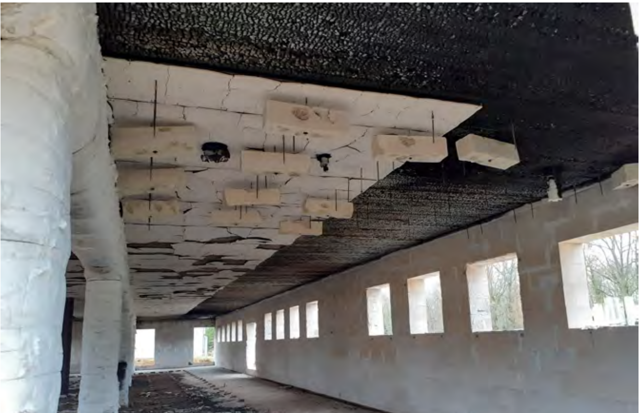
Figure 11. Photo from experiment four, showing extensive external flaming from openings at one end of the building, as the fire reaches the end of the compartment 34 minutes after ignition. Wooden crib at the ignition end of the compartment has largely burnt out already.
