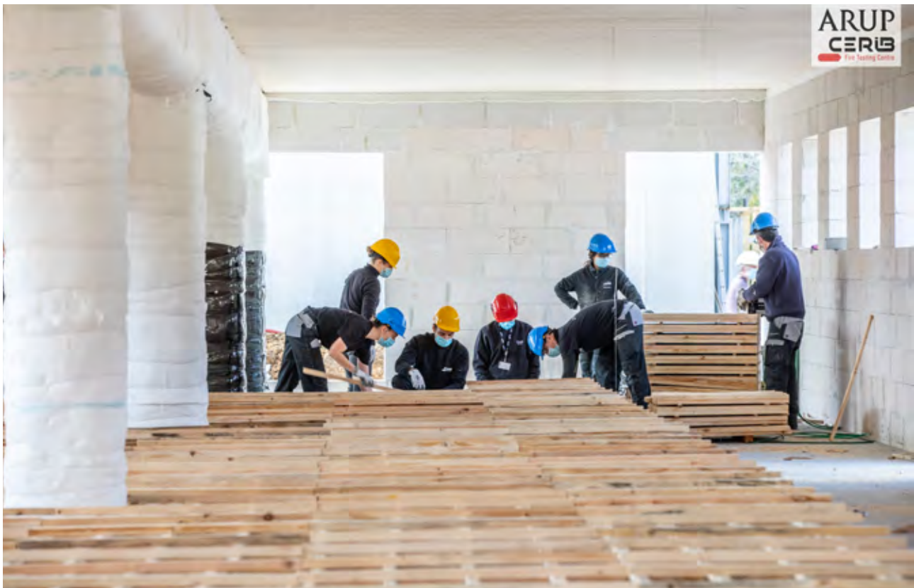
Figure 1. The purpose-built facility 11m wide, 35m long and 3m in height, shown set up for Experiment one. The team are stacking the fuel crib within the compartment to exact specifications.
