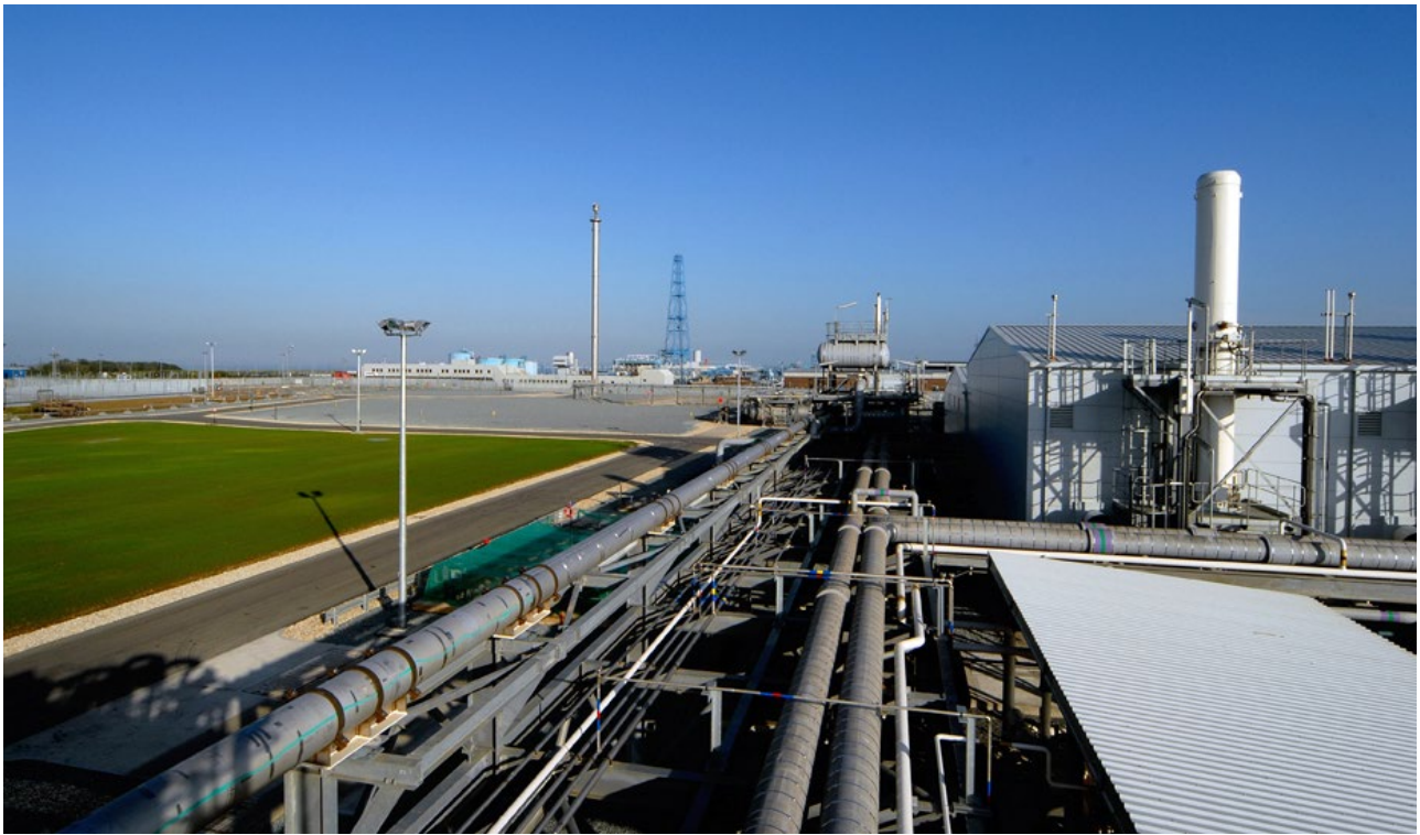
Figure 61: Easington Receiving Terminal (© Gassco)
